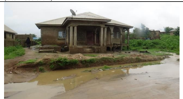
Abandoned structure as a result of flood events
