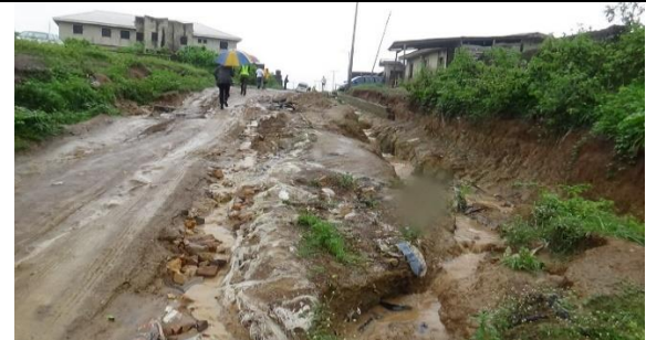
Weathering of top soil as a result of water erosion (after flood event)
